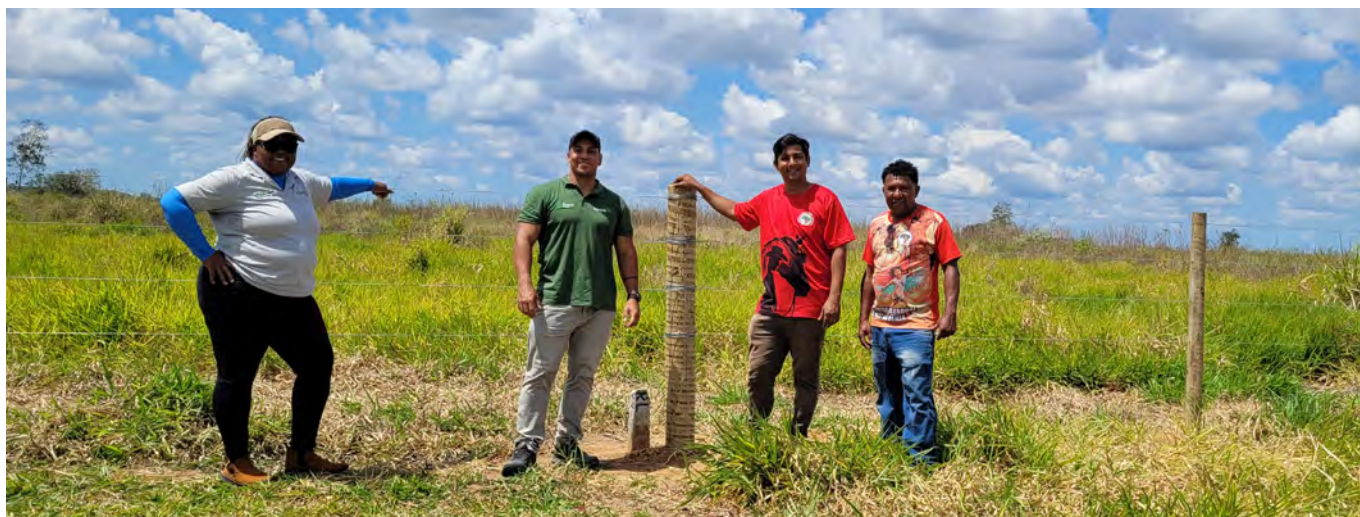
Figure 8. Construction of a fence to delineate and protect the planting area in the Fábio Santos Project.
